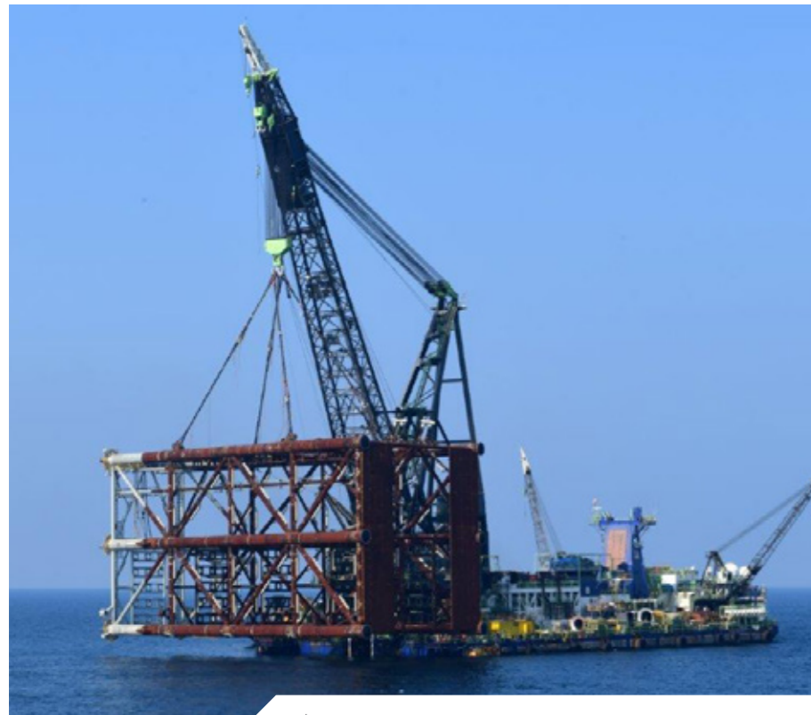
The North Field East (NFE) Expansion Project jacket installation in progress in October 2020.
